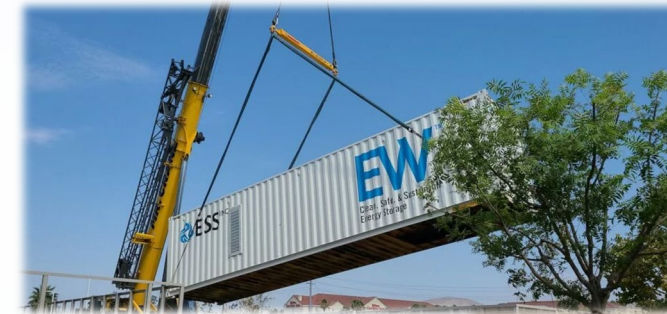
Flow battery storage
